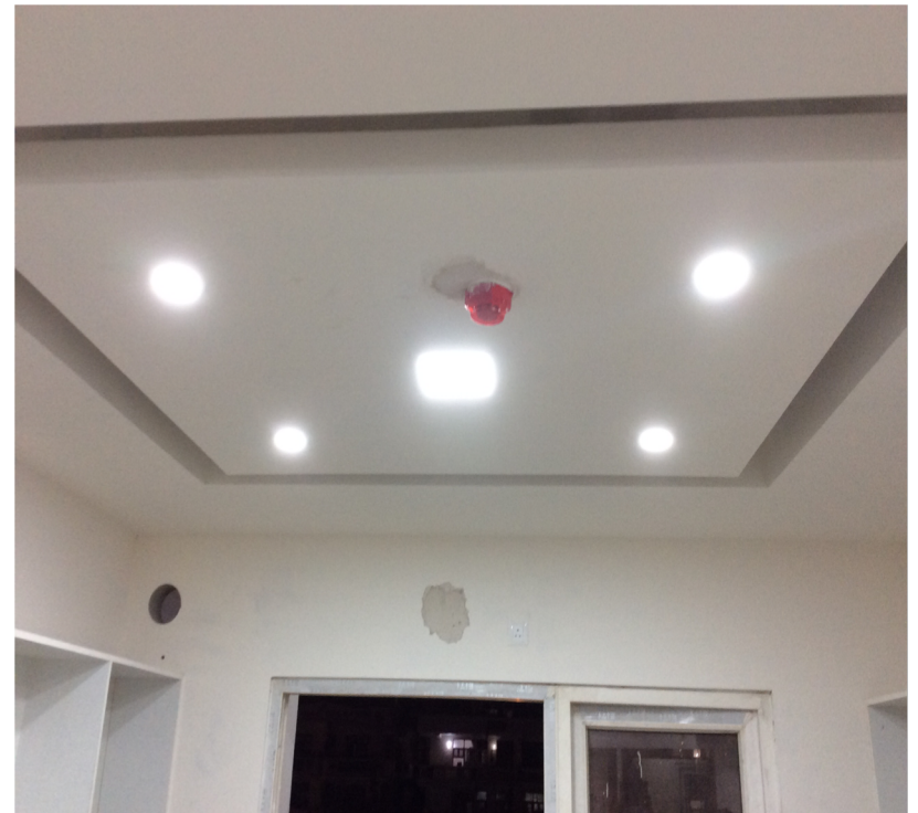
Flats with LED installations
