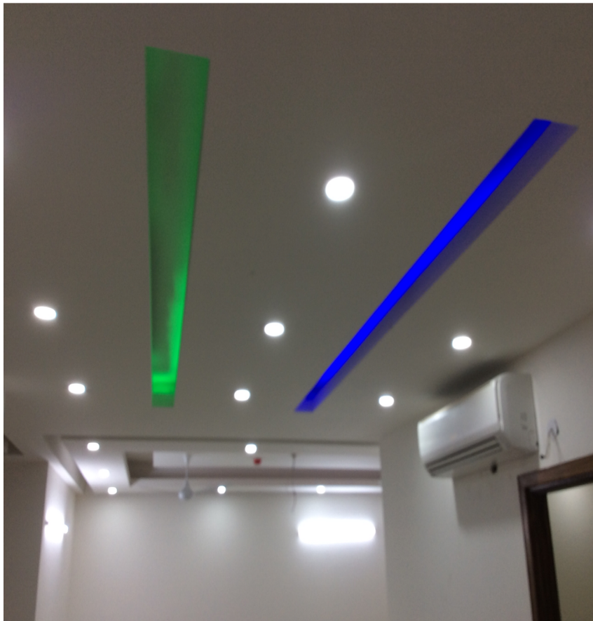
Flats with LED installations
